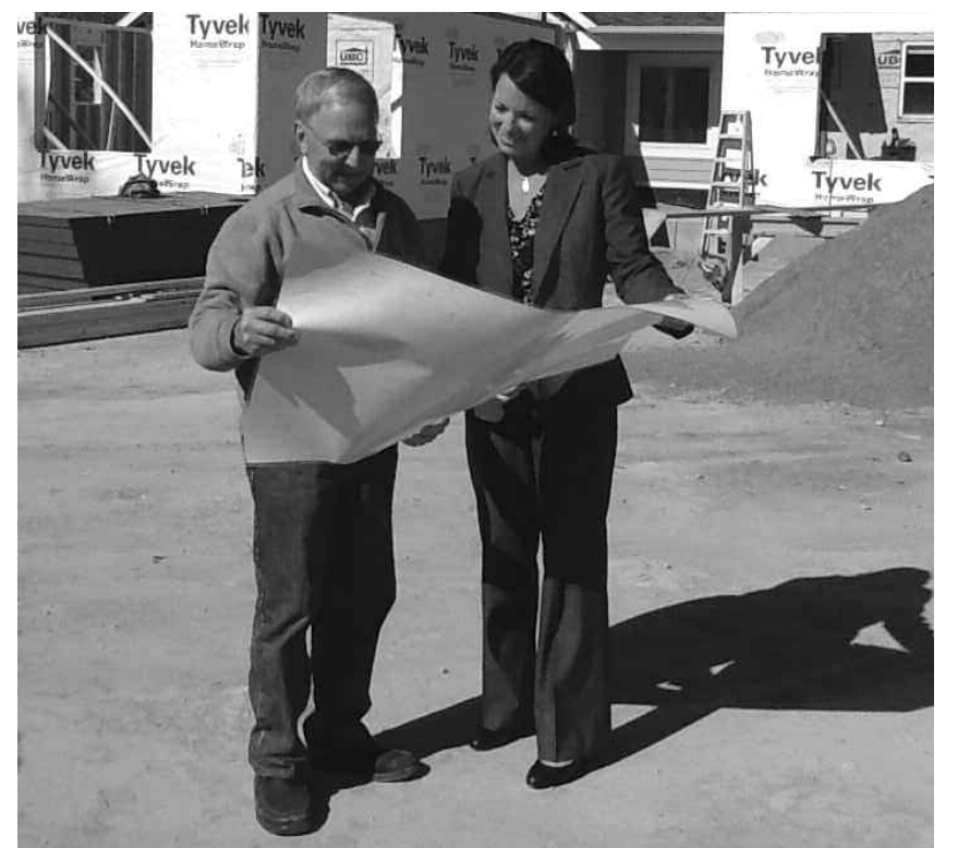
Valerie Snyder, Chair of the Board of Trustees, takes a look at the drawings, and the progress made on the construction for the new facility for the Charlevoix County Community Foundation with Floyd Wright, General Contractor.
